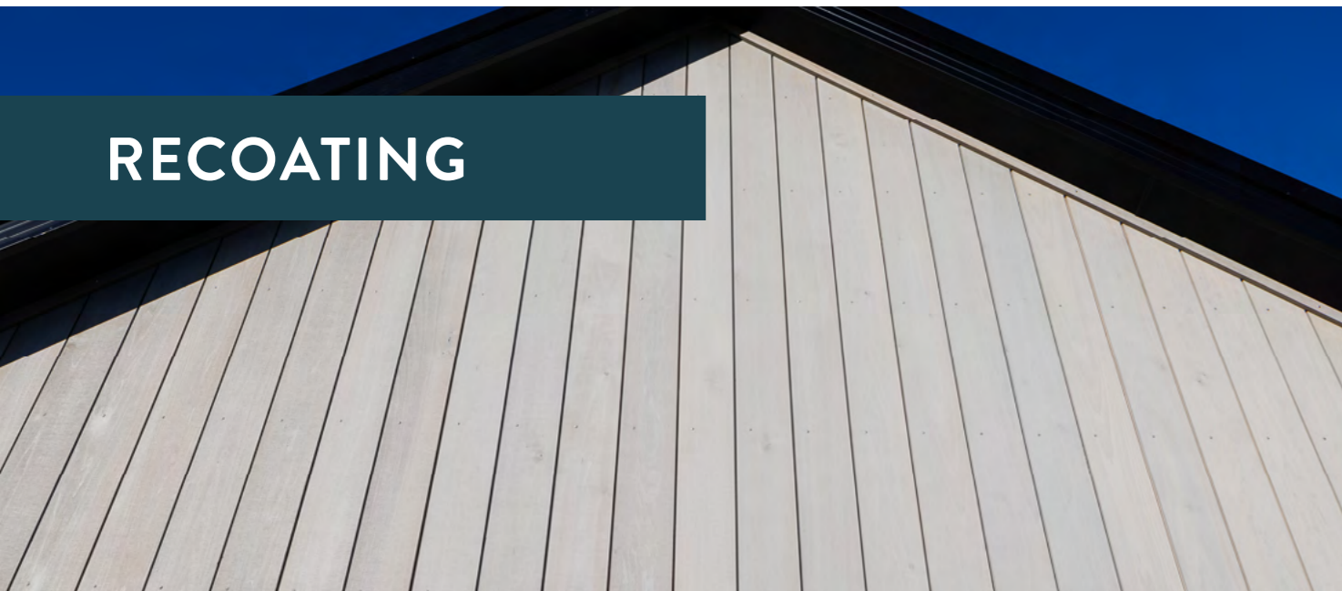
TMT Taxon Vertical Shiplap Weatherboards coated in JSC Scumble® colour Ash Generations Showhome | Taupo
